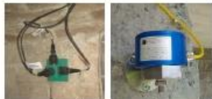
Structural engineering - accelerometers, Heave and settlement monitoring system
